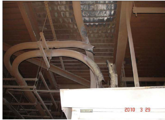
Conduit for electrical cables damaged by the fire at the HB Robinson plant. NRC photo.
