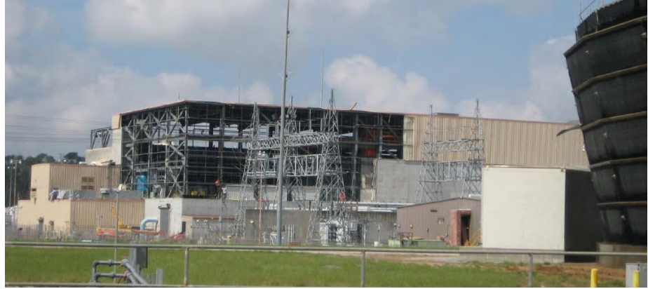
The turbine building at the River Bend plant after Hurricane Gustav removed its metal siding. NRC photo.
