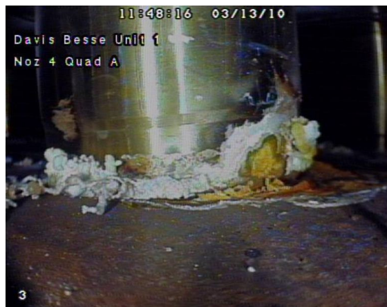
White-crystalline boric acid leaked through a cracked nozzle in the head of the reactor vessel at the Davis-Besse plant in Ohio. NRC photo.
